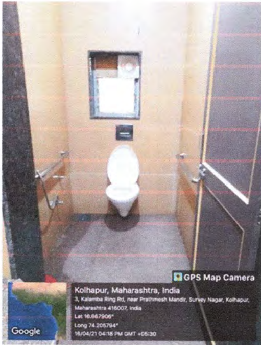
Ramp Facility in Toilets
