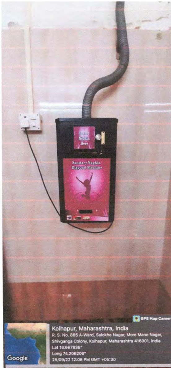
Sanitary Pads Incinerator
