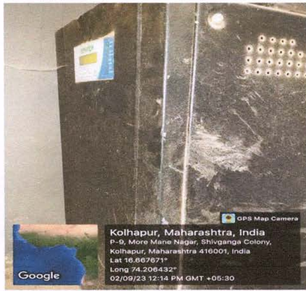
7.5 kVA UPS system
