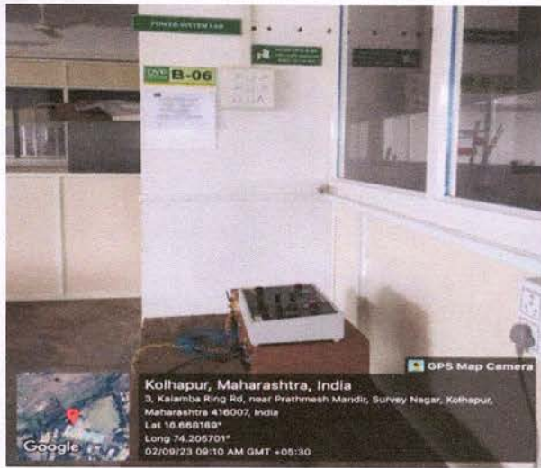
Basic Electrical Engg. Lab
