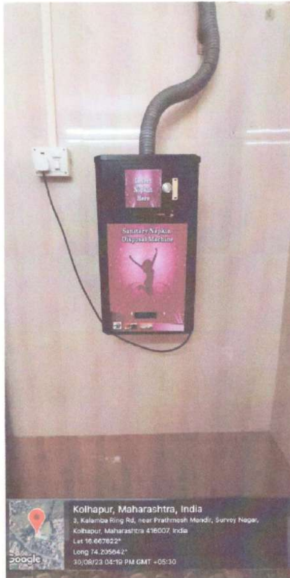
Sanitary Pads Incinerator
