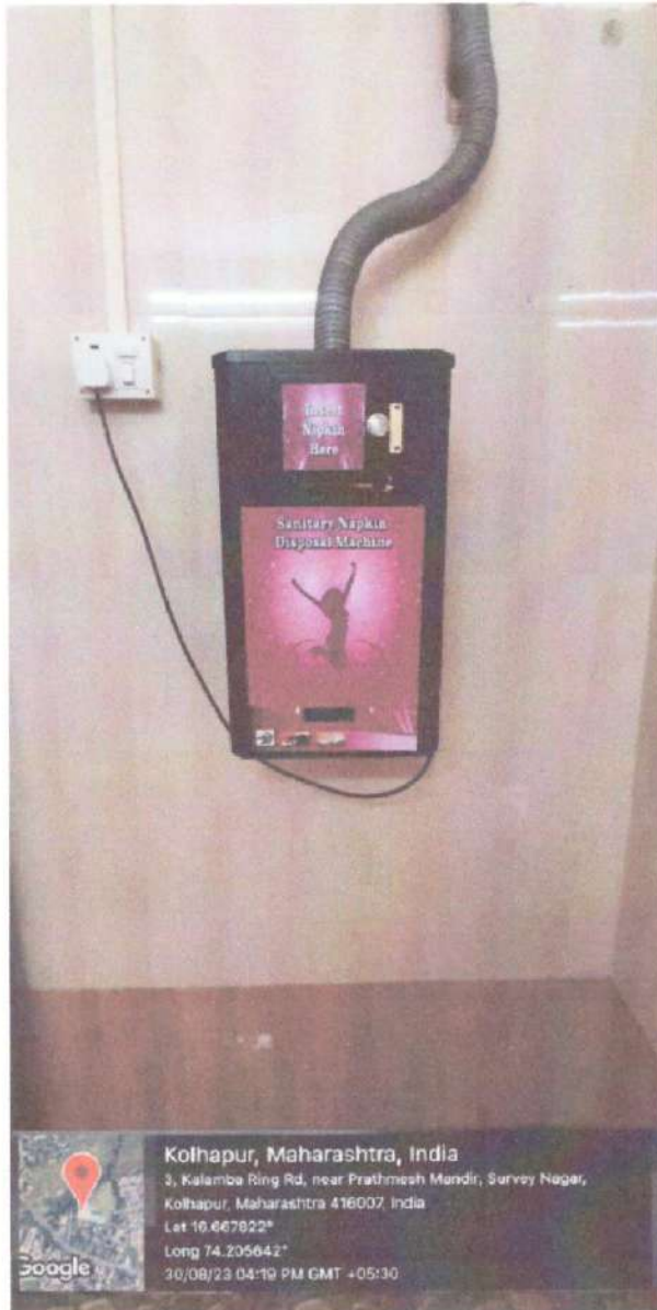
Sanitary Pads Incinerator
