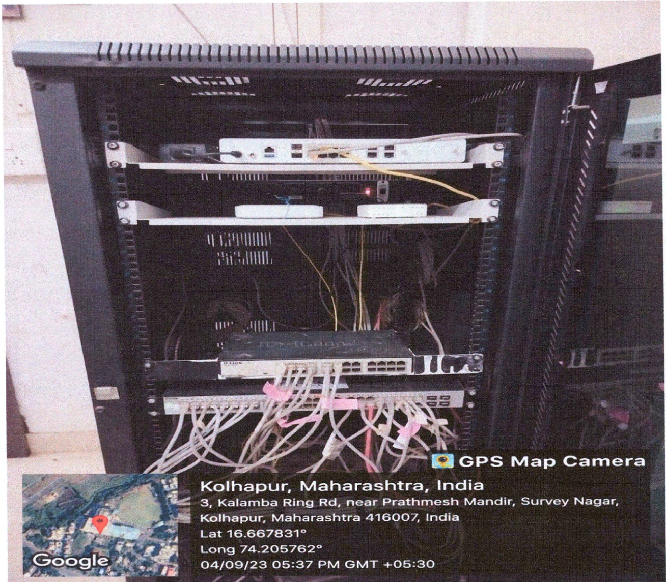
Loaded Server Room Rack
